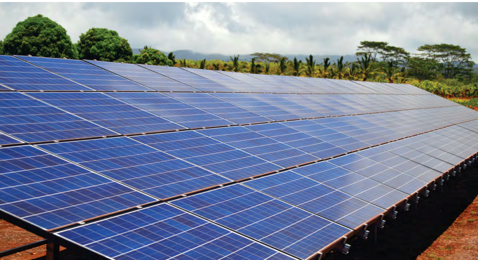
A long row of solar panels is installed in an open field in Hawai'i. © kirkikis / iStock
